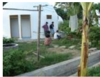
Figure 3. Gotong royong making plumbing & a new well around an MCK. Source: Field survey.
